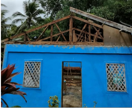
Storm Damage to the Church Building
